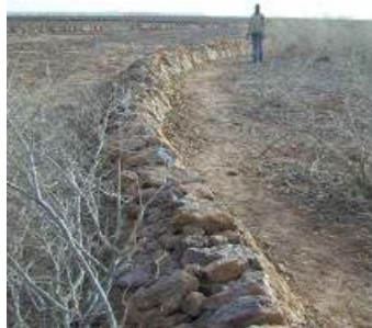
Correctly built Contour Rock Wall Terraces (CRWTs) at Gabda Fandou, Tillabéri South, March 2014. These terraces, built on slopes of the escarpments, significantly retard run off, stop gullyng, and improve aquifer recharge.
