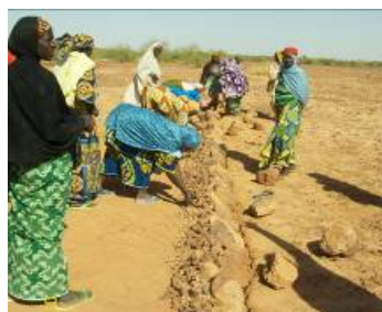
Women construct contour stone bunds at Sourgo Koira Village, Tillabéri South, Feb. 2014. These previously landless women now have land where they will plant hardy vegetables. The bunds harvest water in significant quantities.
