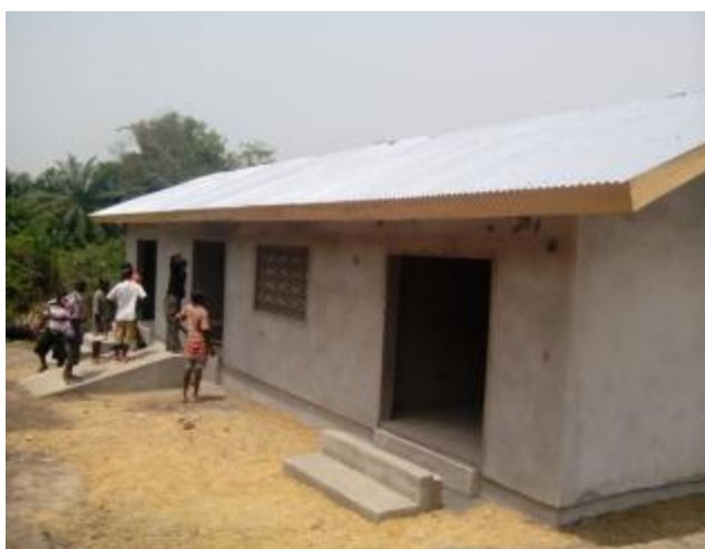
Figure 2: The rice processing center in Payee, Nimba county, has a roof and is ready to receive a processor.
