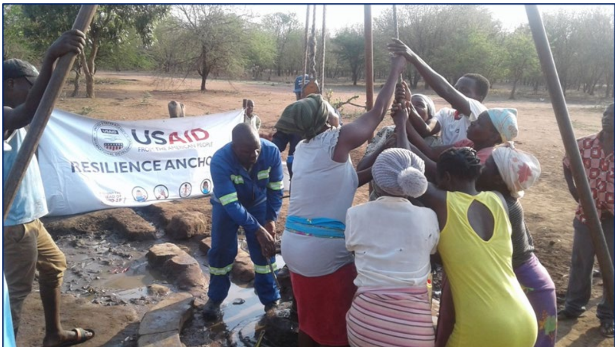
Figure 13: The DDF carrying out the borehole capacity test for the village 2 borehole in Nyangambe, Chiredzi with community participation
